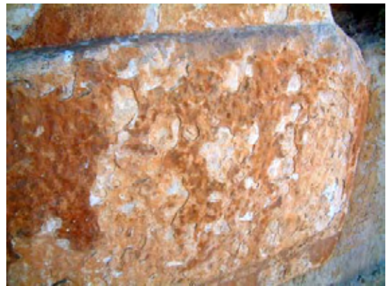
Destructive agents at work on Stone-built monuments
